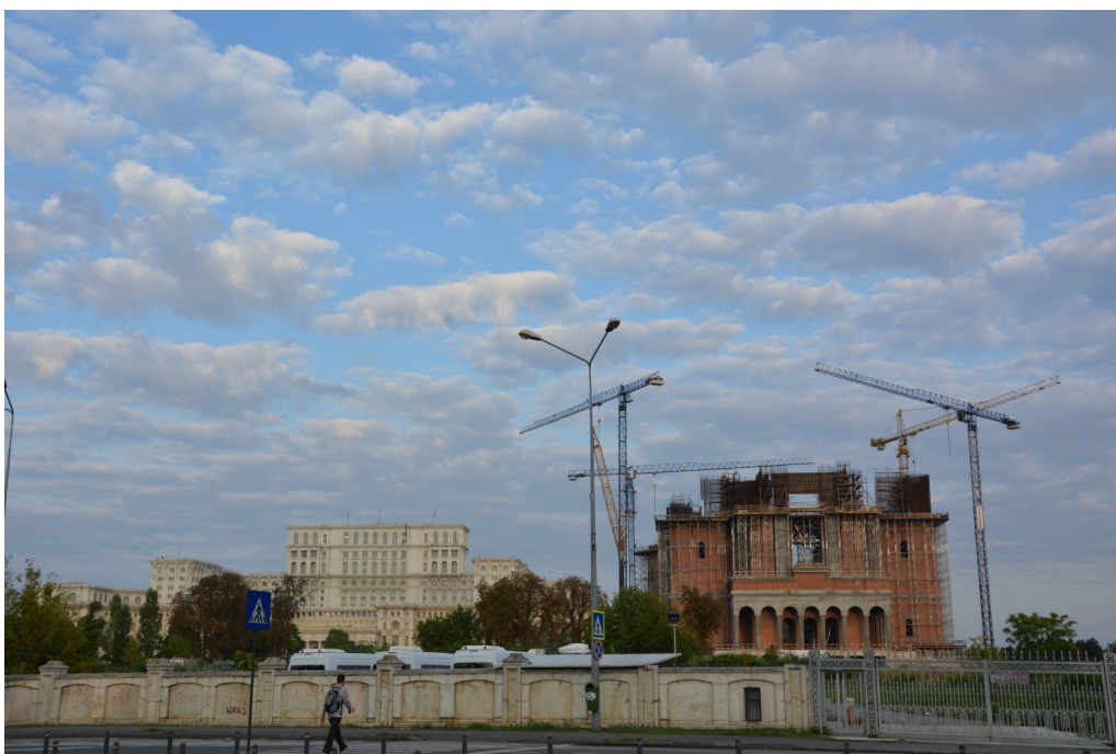
FIG. 1: The Cathedral for the Salvation of the Romanian People on construction. In the background, the Palace of the Parliament.
